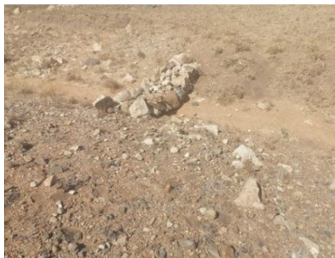
Using stone packs and wattle branches to restore degraded land and promote sustainable grazing practices
